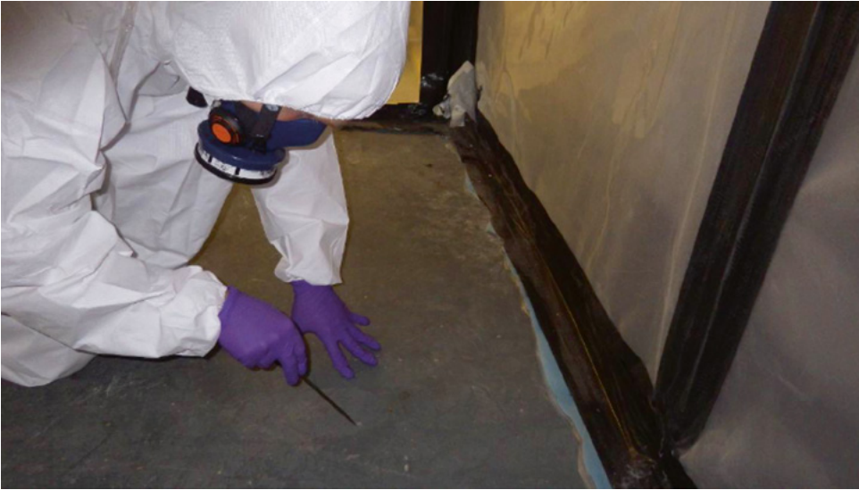
Figure 6.3 Analyst using a screwdriver to check for remnants of asbestos
