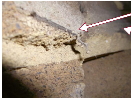
Figure A5.9 Remnants of asbestos on materials
